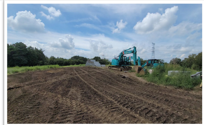
→ Site of Nasu Karasuyama Solar Power Plant
