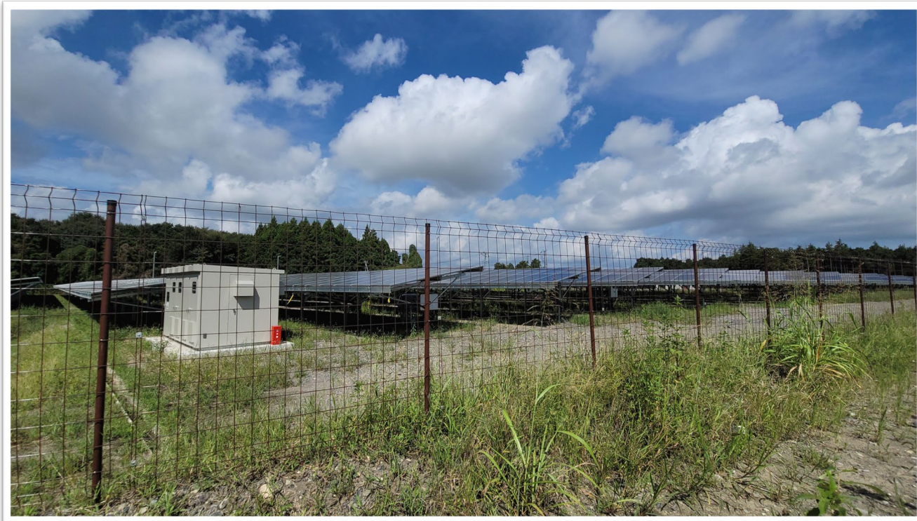
↑ Kami Ishikawa Solar Power Plant
