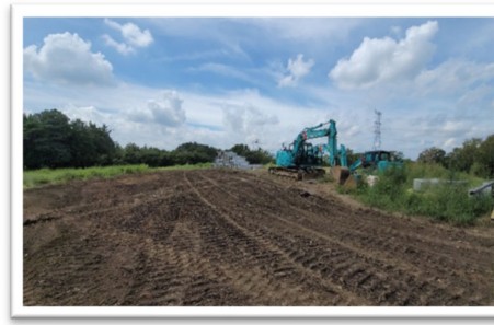
Site of Nasu Karasuyama Solar Power Plant
