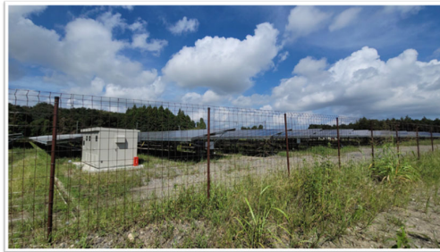
Kami Ishikawa Solar Power Plant
